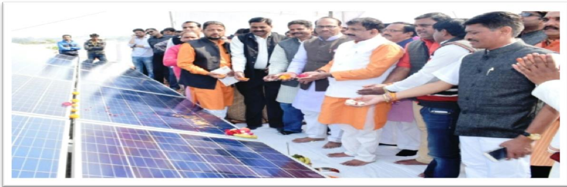
1Mw Solar power plant installation is in progress on Upper lake front beside VIP road
